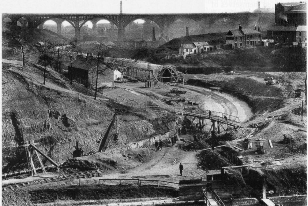
Construction of the Ouseburn culvert in 1907 – this is the lower end of the culvert beneath the Byker bridges and shows the massive scale of the project.
